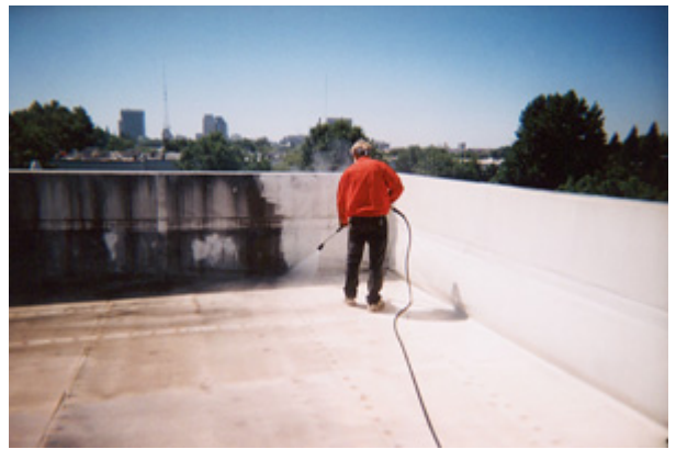
Power washing with hot water to remove algae from the existing PVC roof
