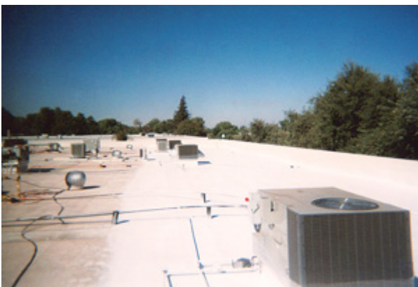
The new reinforced coating system in the process of being applied over the old PVC membrane
